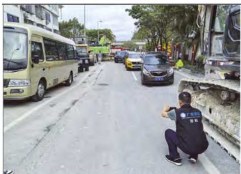
图3 5月18日上午倾斜变形的柳太路路面 Fig.3 Inclined and deformed pavement along Liutai Road on the morning of May 18
