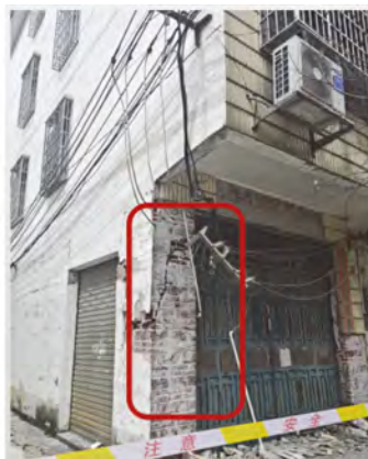
图5 由于地基受到沉降引起砖柱发生断裂破坏,造成房屋严重破坏 Fig.5 Severe building damage induced by brick column fracture due to foundation subsidence
